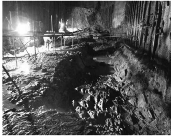
Fig. 2 Zone of crushed weak rock in the left dam abutment of Jinping I [12].
